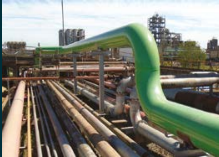
New pipeline at GS Inima Industrial Triunfo.
